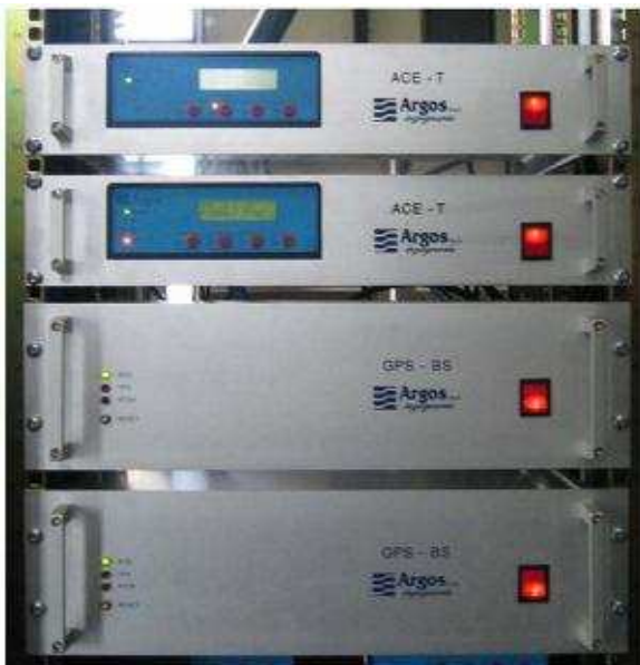
Figure 7: Ground Station Equipment
